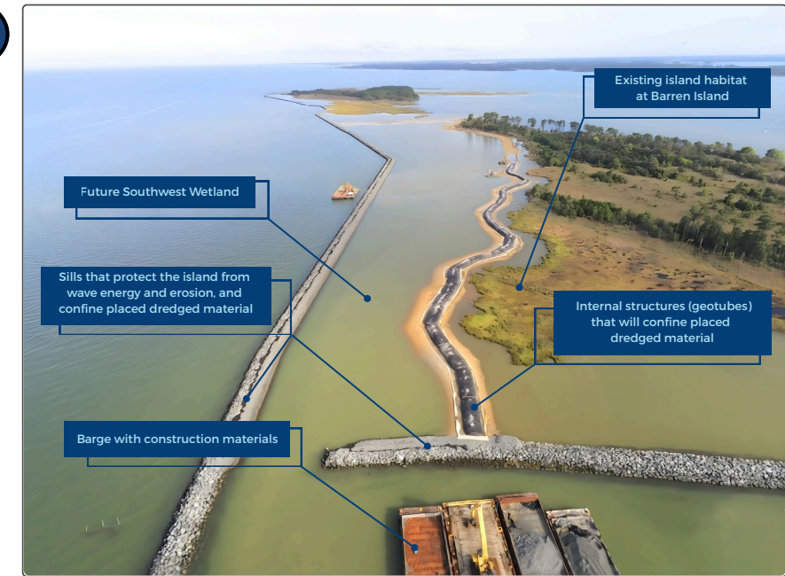
Figure 2. A birds-eye view of construction progress at Barren Island. Photo courtesy of GBA in September 2025.
